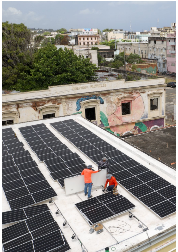
Solar panels being installed as part of the Community Energy Resilience Initiative in Puerto Rico | Credit: RMI
